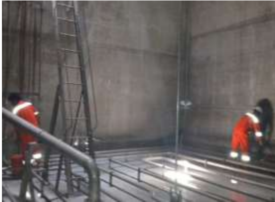
Figure 3. Cargo Residue on Loading Tanks
