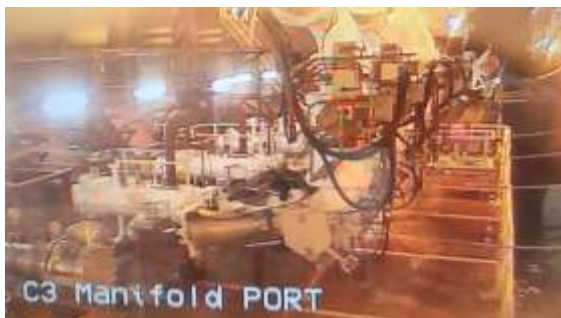
Figure 3. Leak in the cooldown valve
