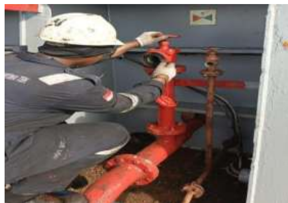
Figure 2. Maintenance Fire Hydrant
