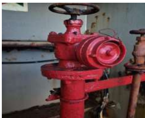
Figure 1. Fire Hydrant has experienced a decline in quality
