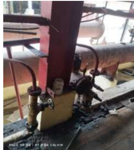
Figure 3. Ammonia Filling Valve
